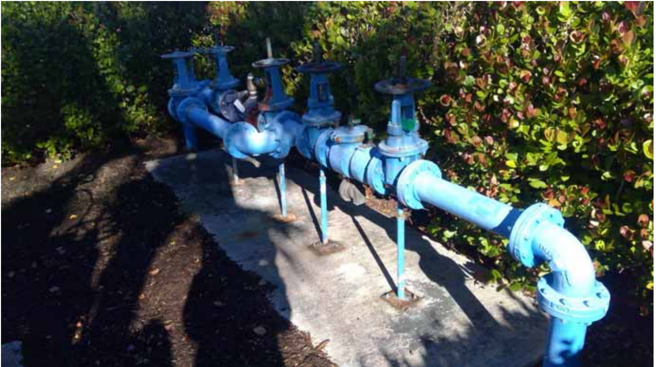
Backflow Preventer - Domestic
