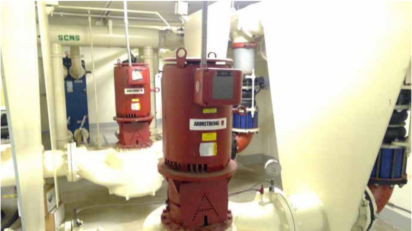
Cooling Tower Pumps
