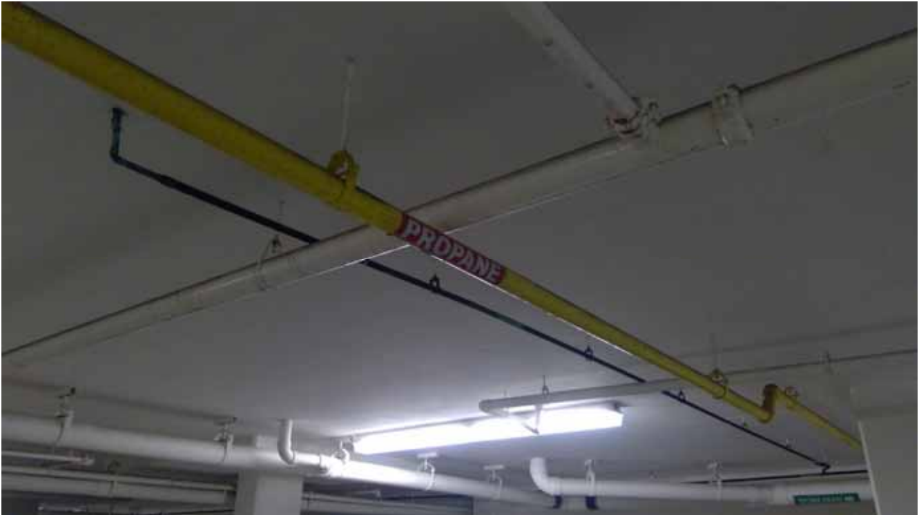
Plumbing Lines - Parking Garage
