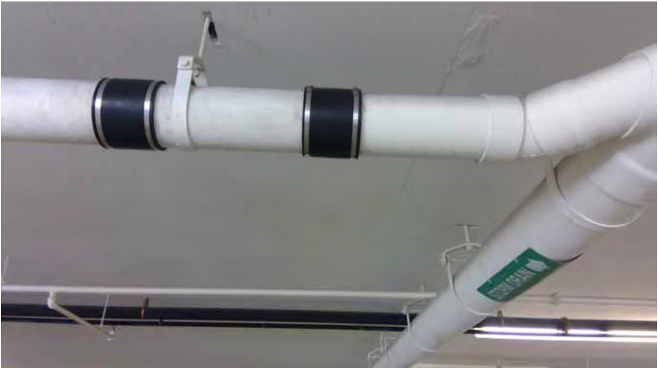
Plumbing Lines - Parking Garage
