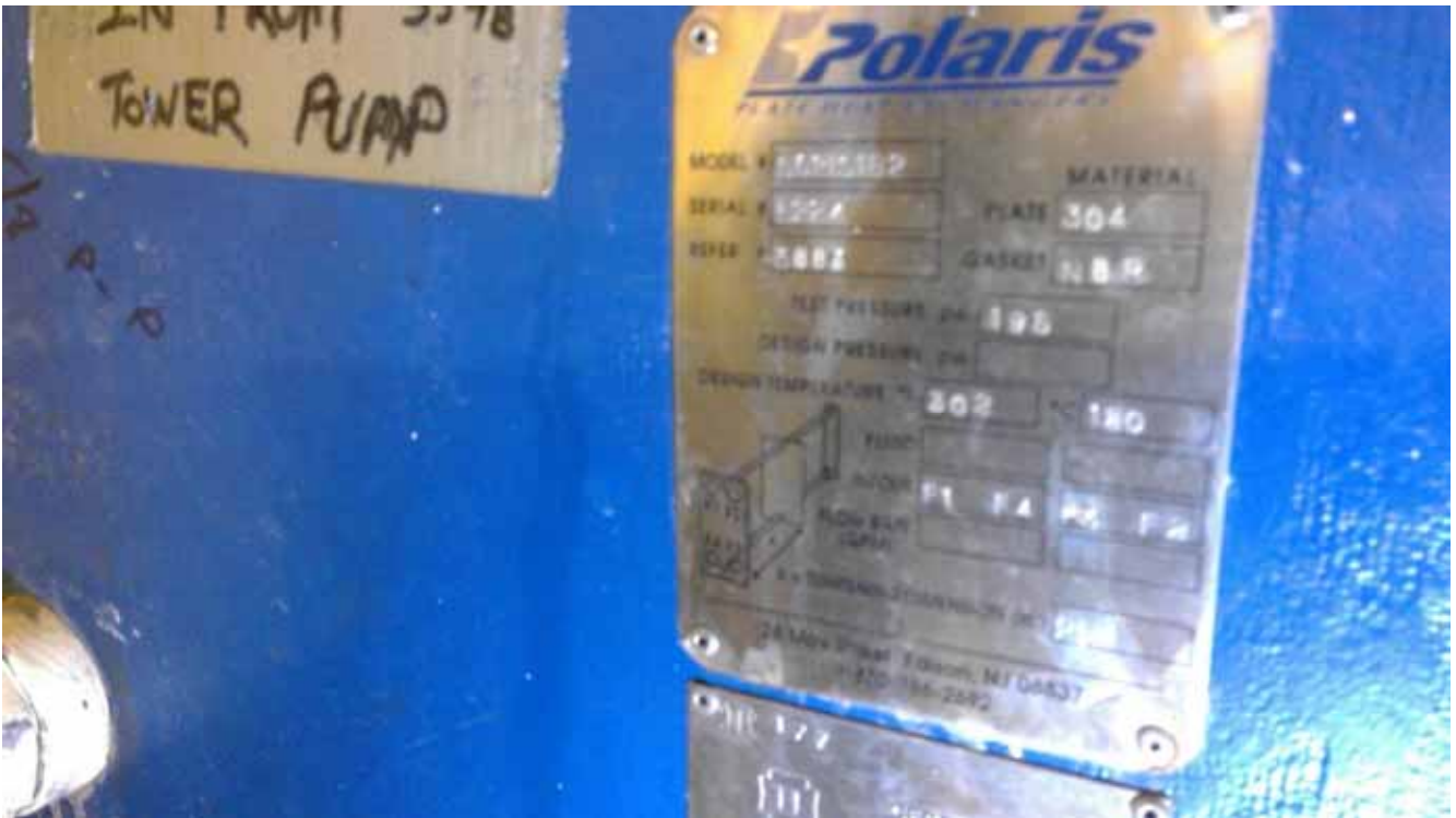
A/C Heat Exchangers
