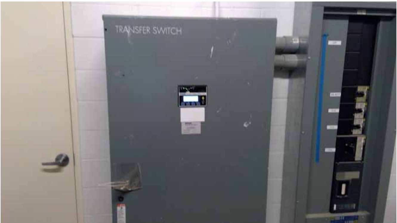
Transfer Switch - Generator
