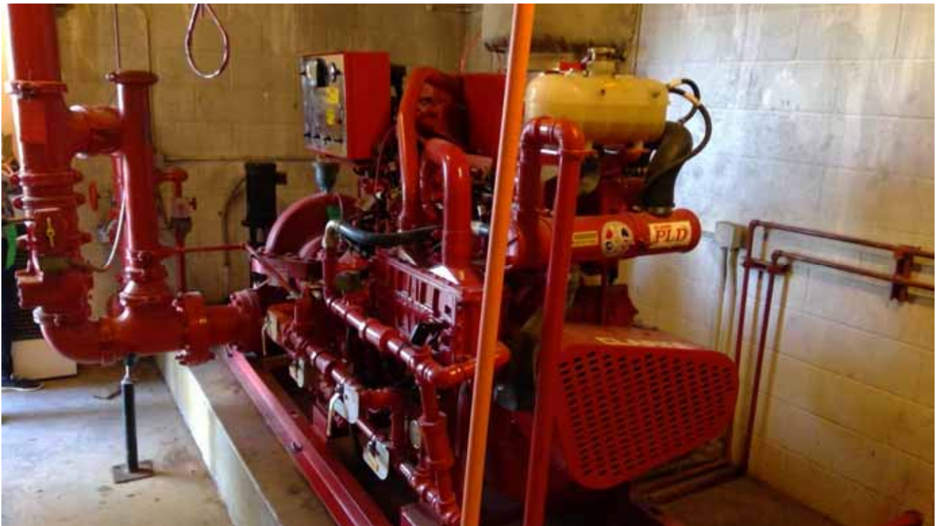
Fire Pump - Diesel
