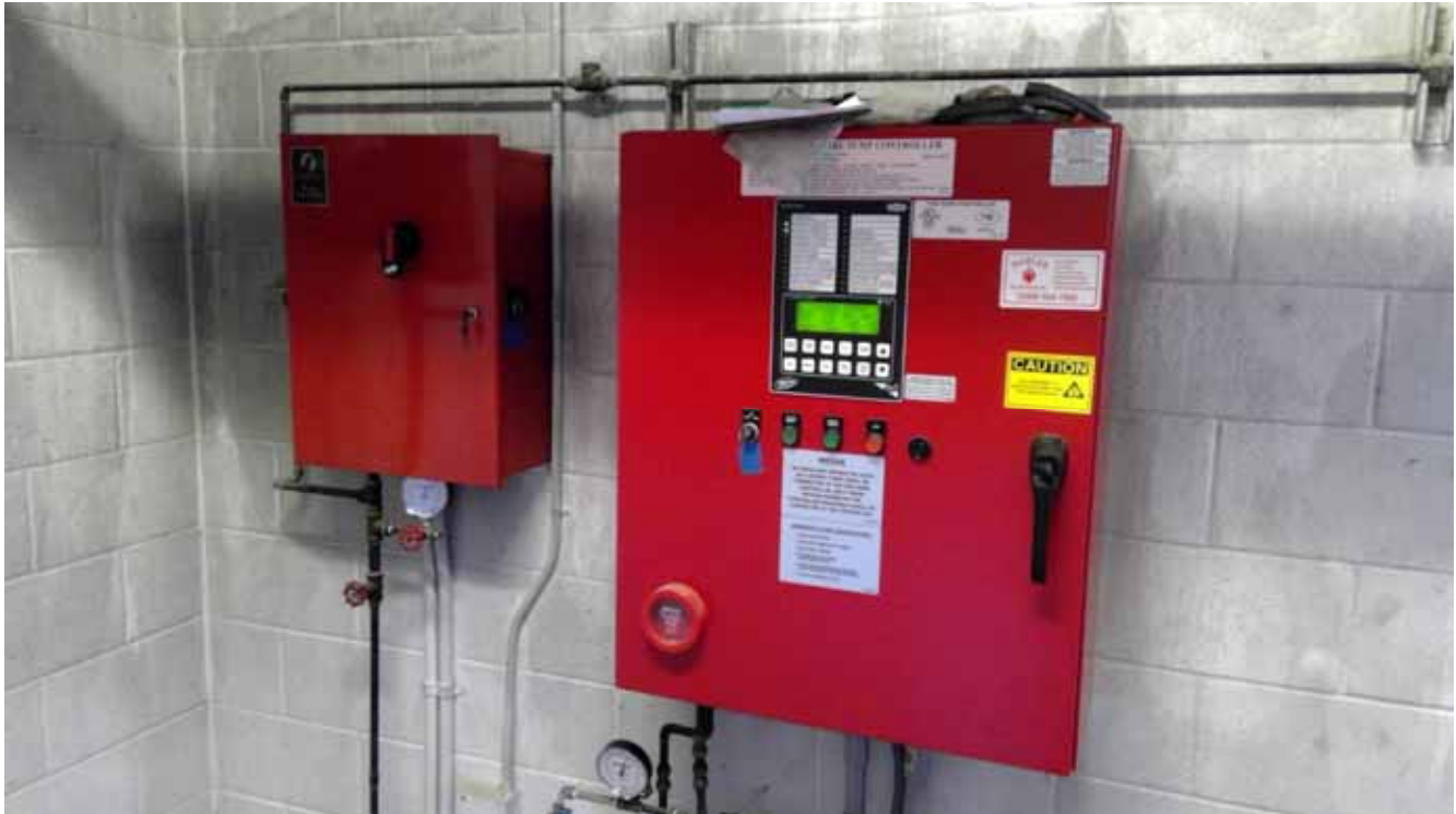
Controller - Fire Pump
