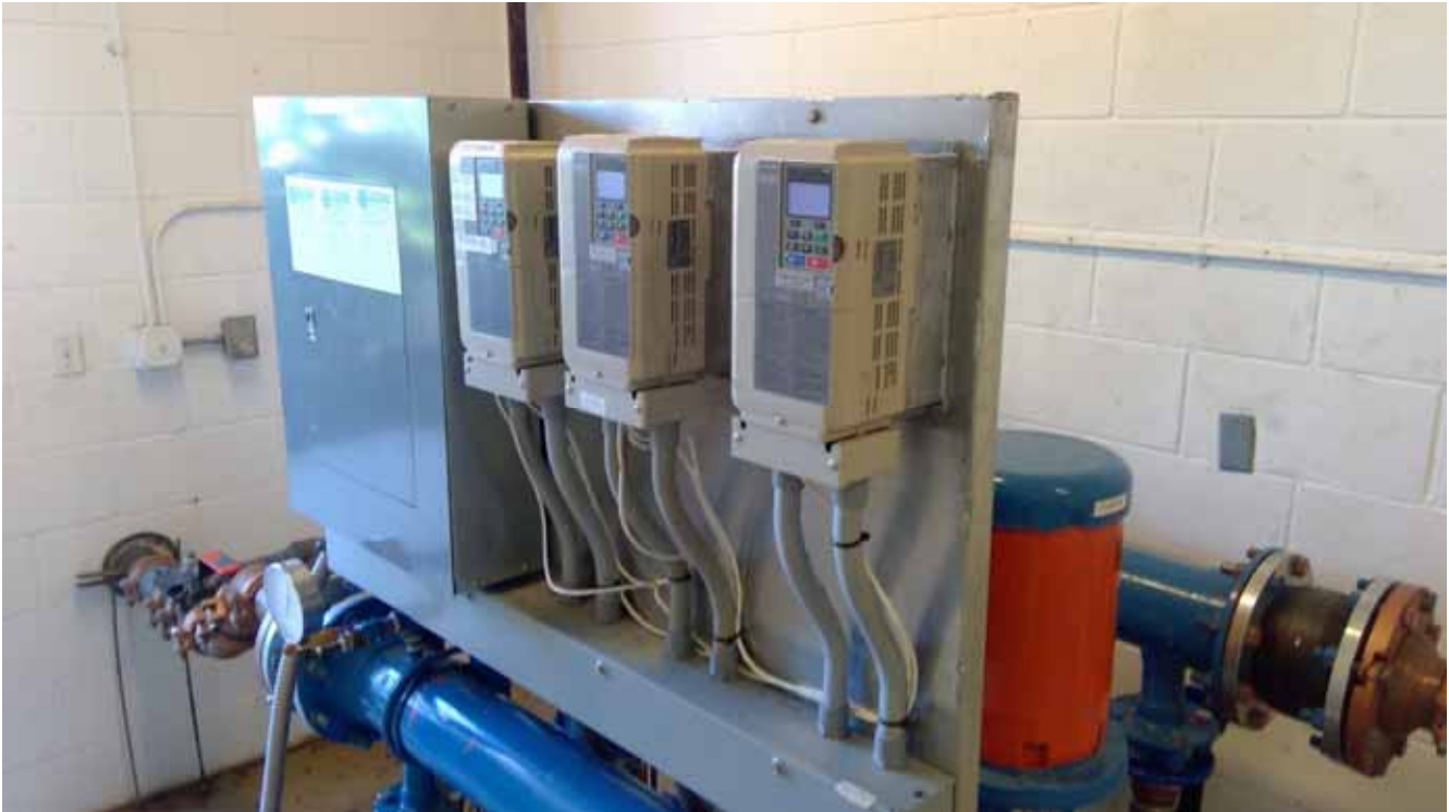
Domestic Water Pumps
