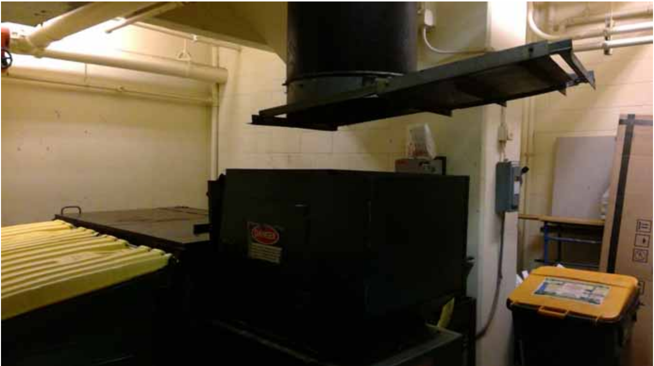
Trash Chute - North
