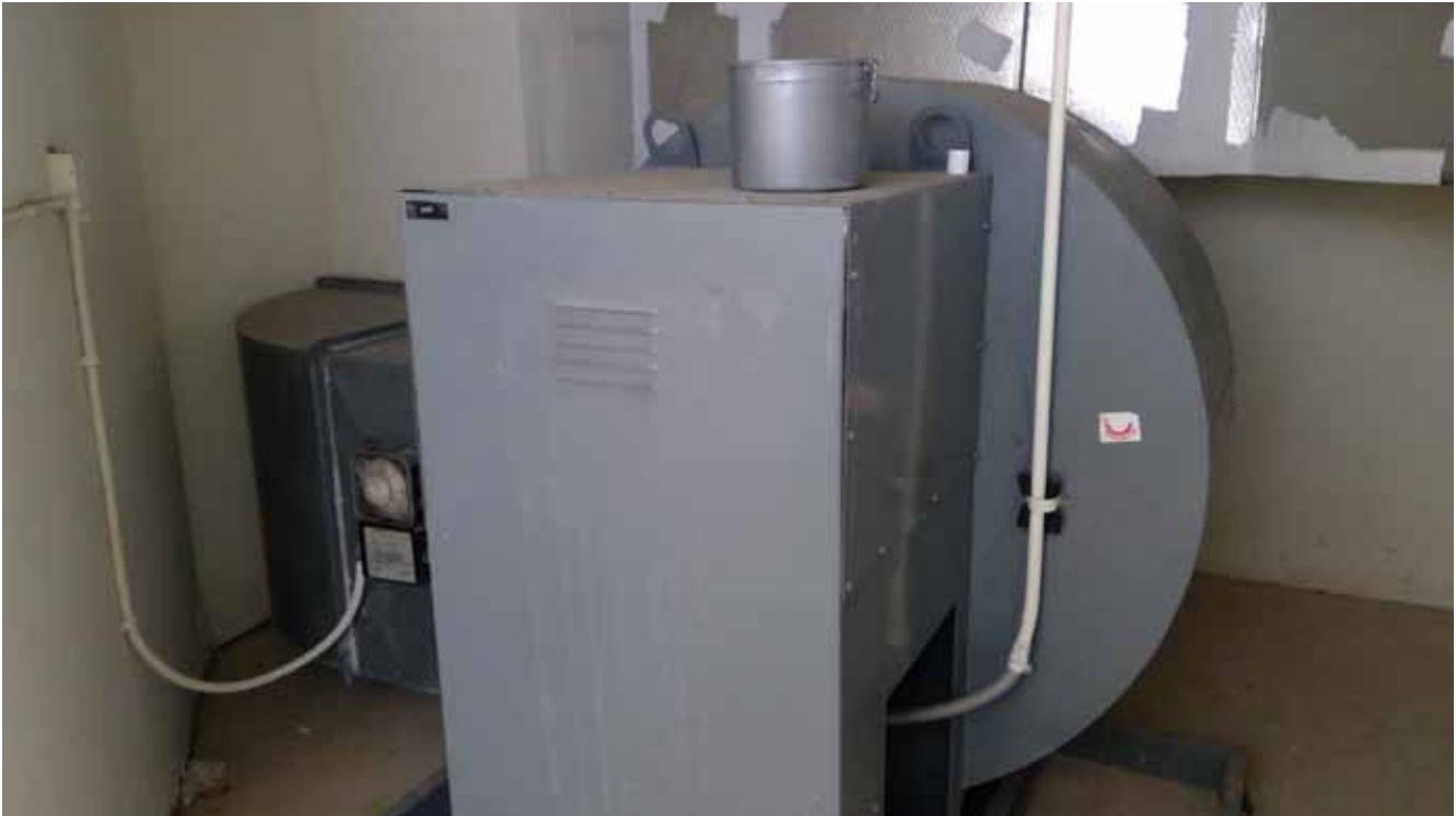
Stairwell Pressurization - South
