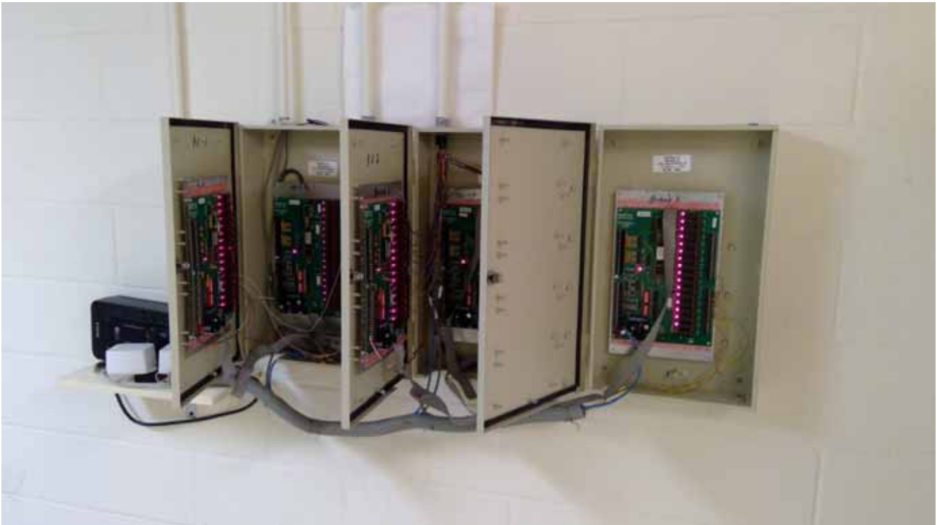
FOB Access Relays - North
