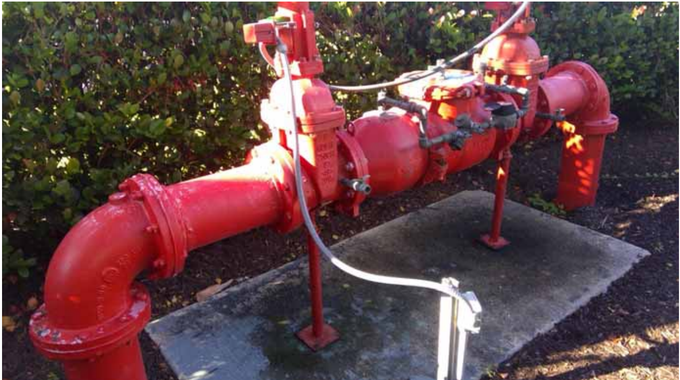
Backflow Preventer - Sprinklers
