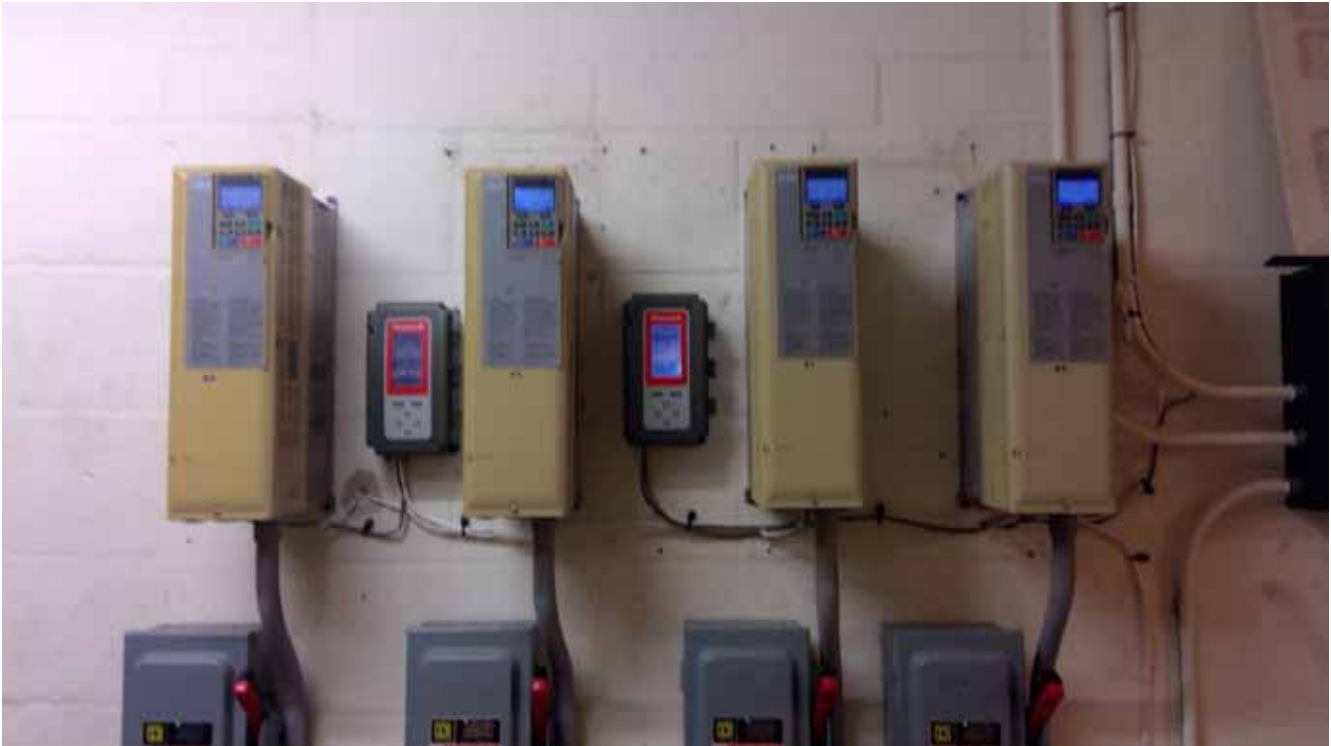
VFD's Cooling Towers
