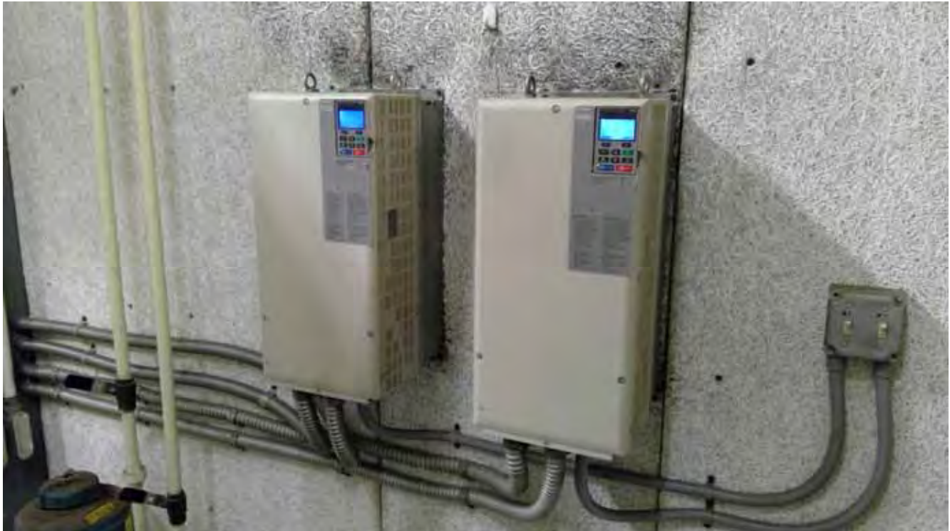
VFD's A/C Circulation Pumps
