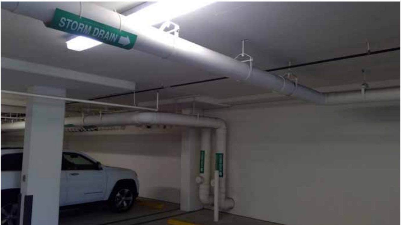
Plumbing Lines - Parking Garage
