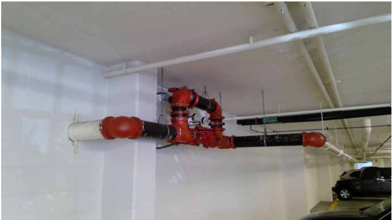
Clay Valve - Fire Sprinklers
