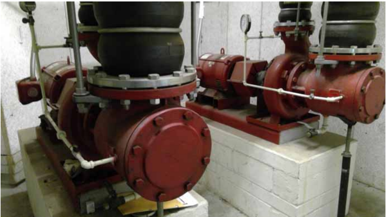
A/C Circulation Pumps
