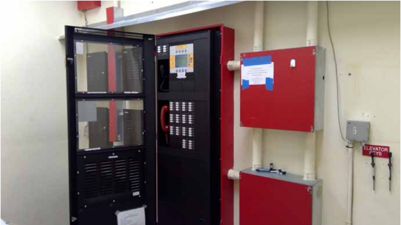
Fire Alarm Control Panel
