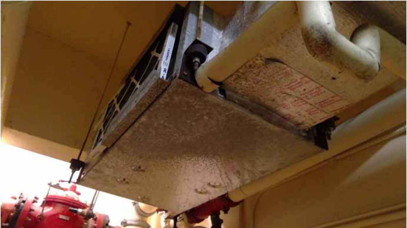
A/C Trash Room - South
