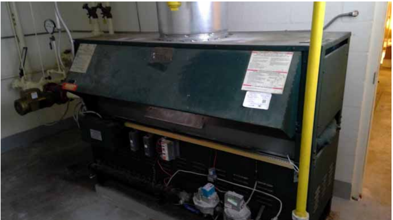
A/C Boiler (Heat)
