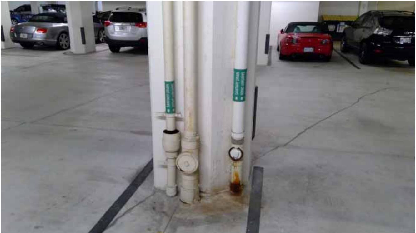
Plumbing Lines - Parking Garage
