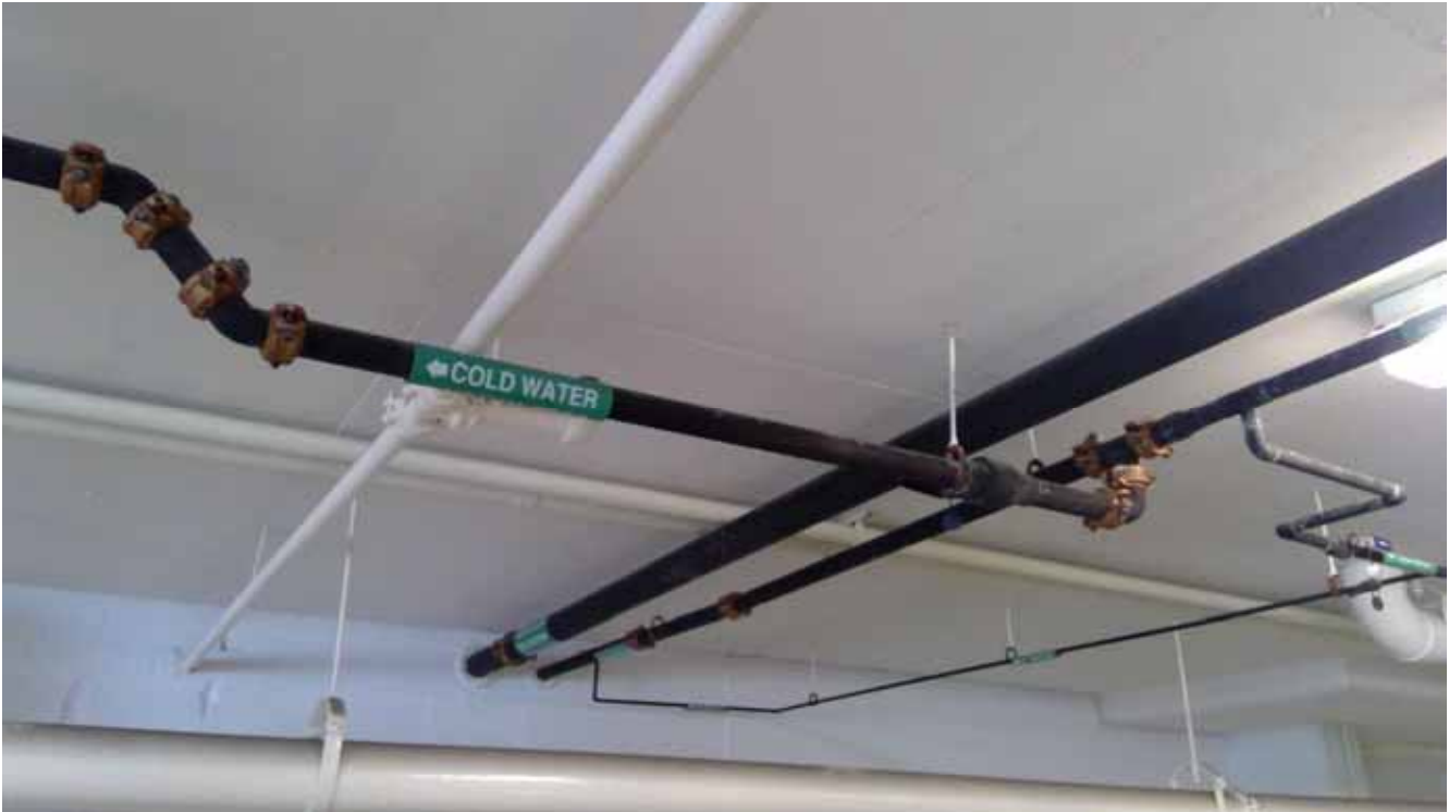
Plumbing Lines - Parking Garage
