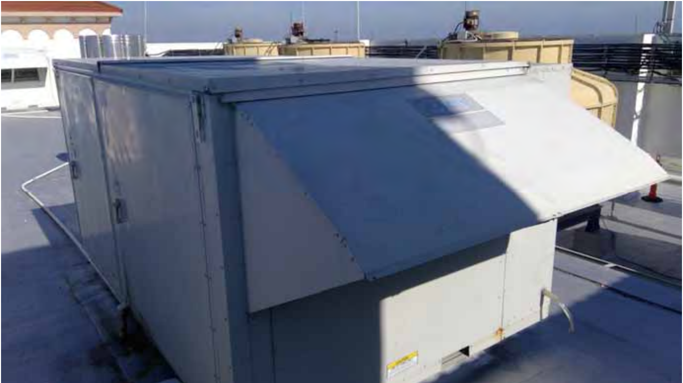
Aaon - RTU Service Halls
