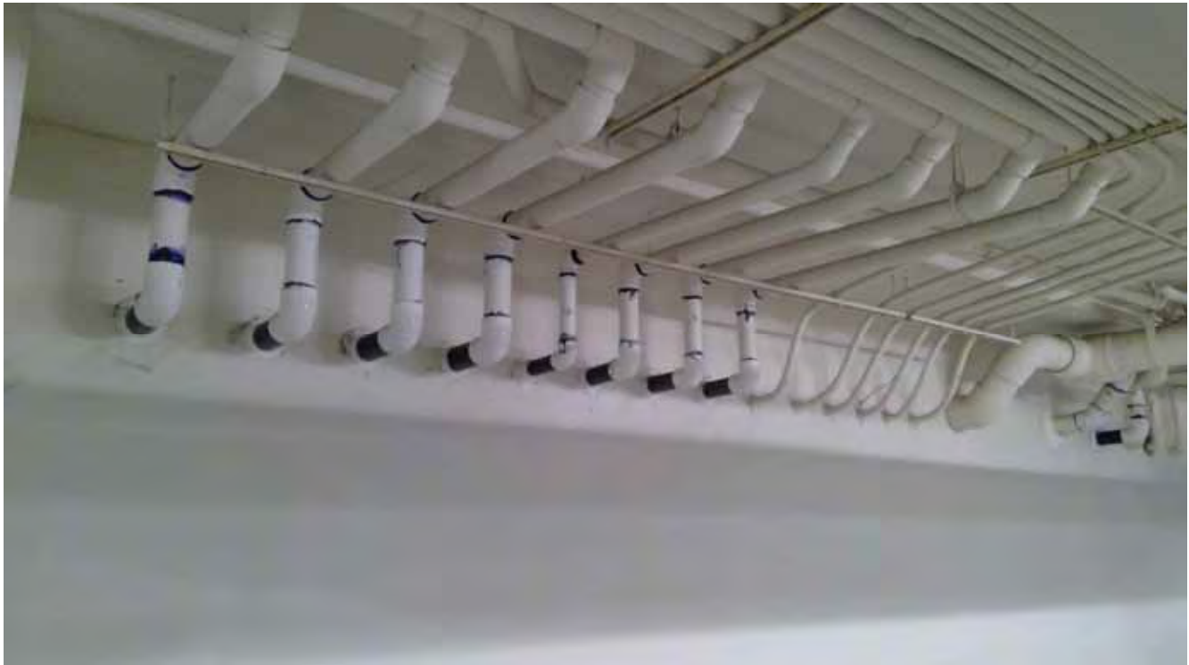
Plumbing Lines - Entry Fountain
