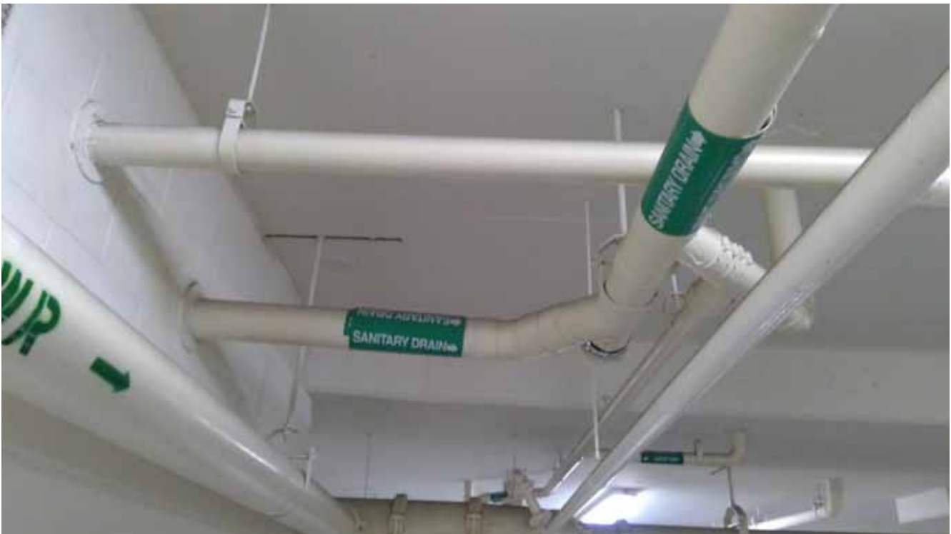
Plumbing Lines - Parking Garage
